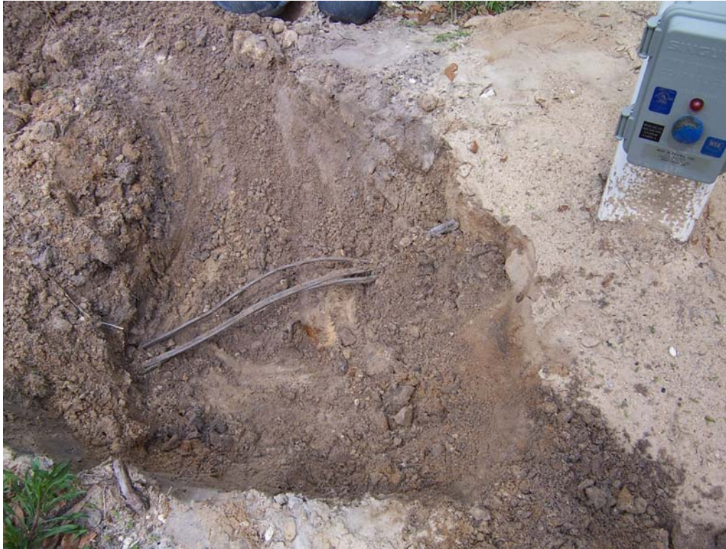
Figure 15. Picture taken on 04/20/09 of Norweco system with wires strung across the pump tank lid preventing access. No sampling port was installed. Maintenance records indicate the effluent was visually inspected.
