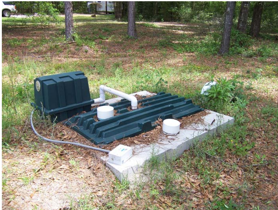
Figure 12. Picture taken on 04/16/09 of a FAST system with the unwired control box lying on the exposed tank. The system was in use with sewage, but no electricity.
