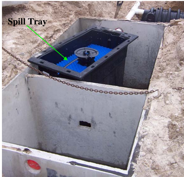
Figure 4. A picture of FAST treatment unit being installed into the treatment chamber of a dual chambered tank. The blue fixed media and spill tray are shown.
